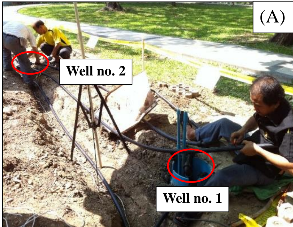
Connecting HDPE pipe of well no.1 to HDPE pipe of well no.2 .
